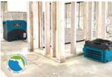
WATER DAMAGE RESTORATION
