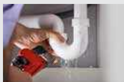
Burst Water Pipe
